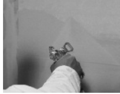
Figure 10c: Spray Sto Gold Coat® or Sto EmeraldCoat® onto the entire wall surface.
