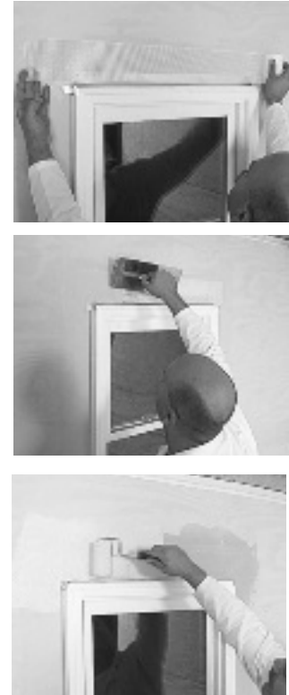
Figure 13: Head Flashing Detail —details like head flashing above windows and doors, roof sidewall step flashing, and starter tracks or flashing at the base of the wall, require a splice strip of reinforcing mesh and Sto Gold Fill® joint treatment, followed by the application of waterproof coating.
